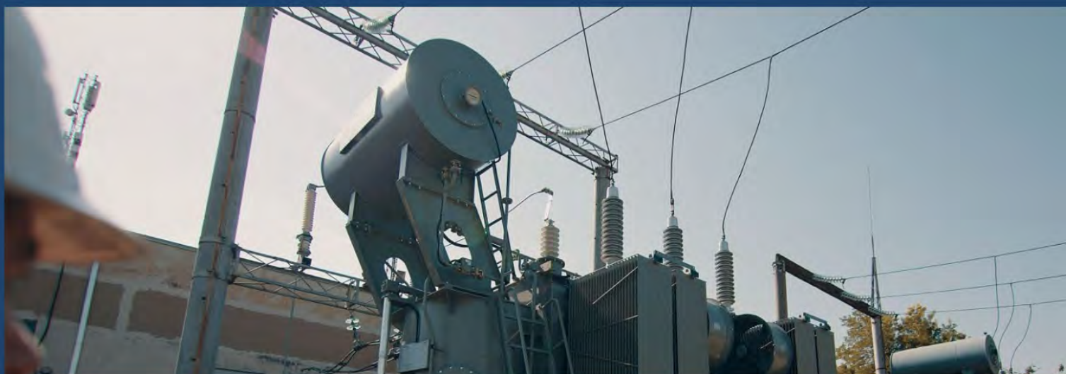
Premier Energy's 110kV Electrical Transformation and Distribution Substation, Valea Trandafirilor, Chisinau, Republic of Moldova
